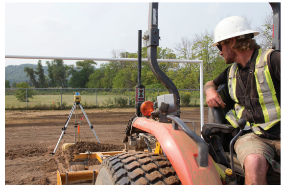
Laser grading sand cap to ensure positive drainage, healthy turf, minimize compaction and improve field durability.
